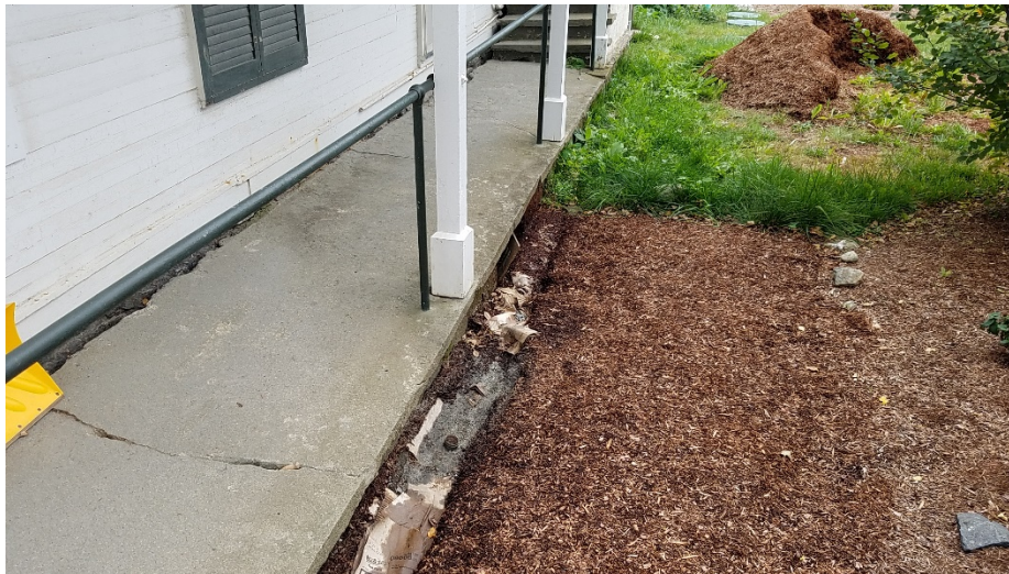
Photograph #6 – Drainage issues directed towards crawlspace access.
