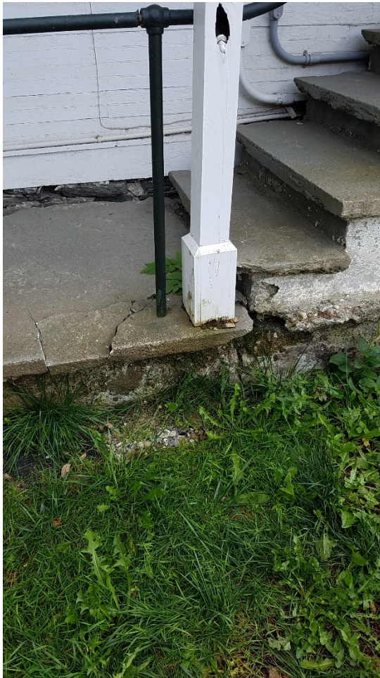
Photograph #2 – Post damage at north porch
