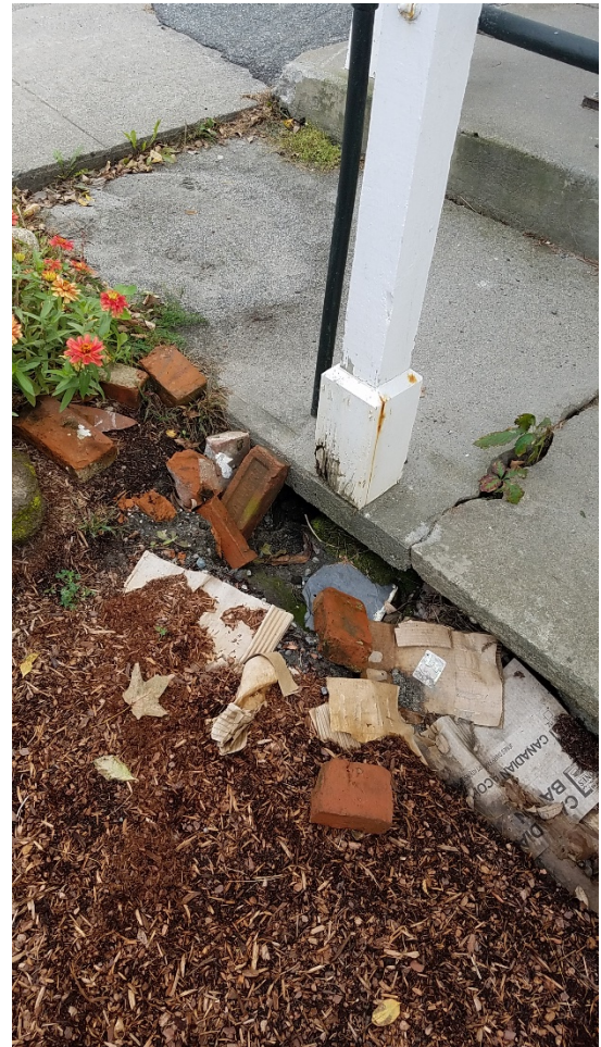
Photograph #3 – Post damage at north porch
