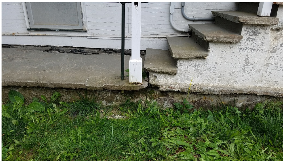
Photograph #7 – Column and north porch support issues
