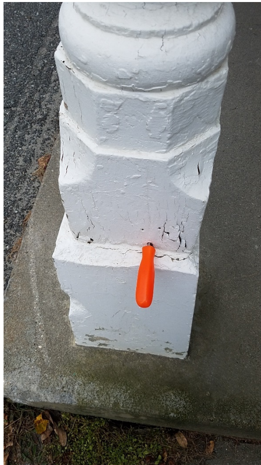
Photograph #1 – Porch post base rot
