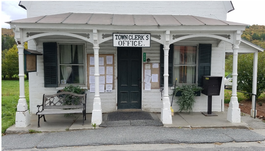
Photograph #5 – Eastern porch movement, eastern sill below grade, drainage towards building/crawlspace.
