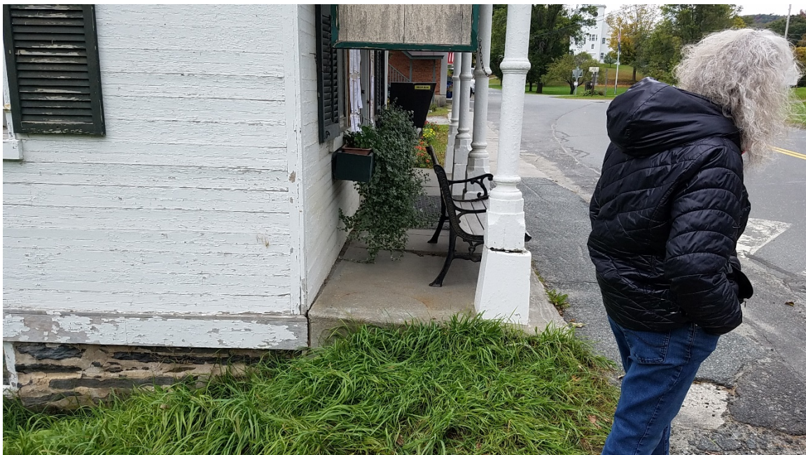
Photograph #4 – Eastern porch slope, pier movement, sill buried in concrete.
